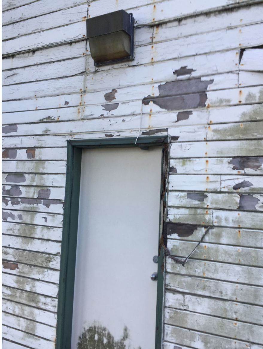
Photo 4: Detail of the east elevation door. The long term preservation plan may include restoring the building's exterior which would restore the original door, window and hay mow openings as well as provide more period appropriate light fixtures with concealed wiring.
