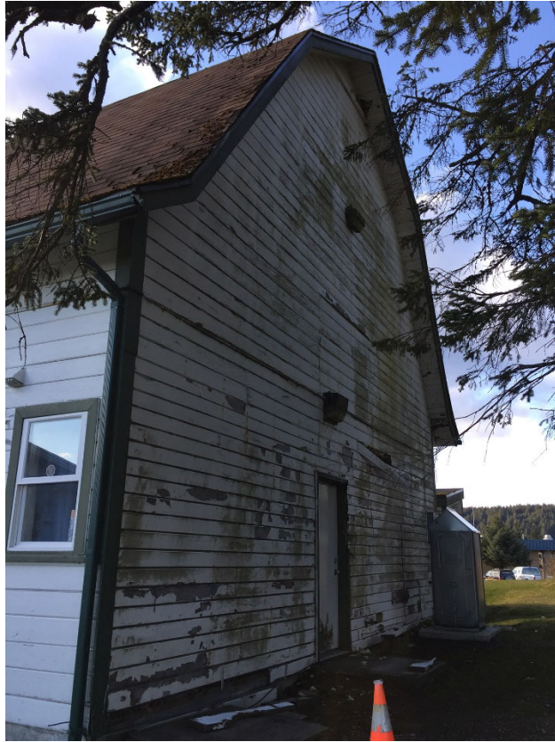
Photo 2: View of the barn’s east elevation. This elevation requires short term stabilization and painting. The evergreen tree is shading this side of the barn and limiting air circulation which prevents the siding from drying – thus the mold. Open siding is permitting wind driven rain into the wall assembly and should be reinstalled as soon as possible in two or more locations on this elevation. Exterior painting for the entire barn is recommended in the near term, next 1-2 years, to ensure the original fabric is not compromised. NPS photo.
