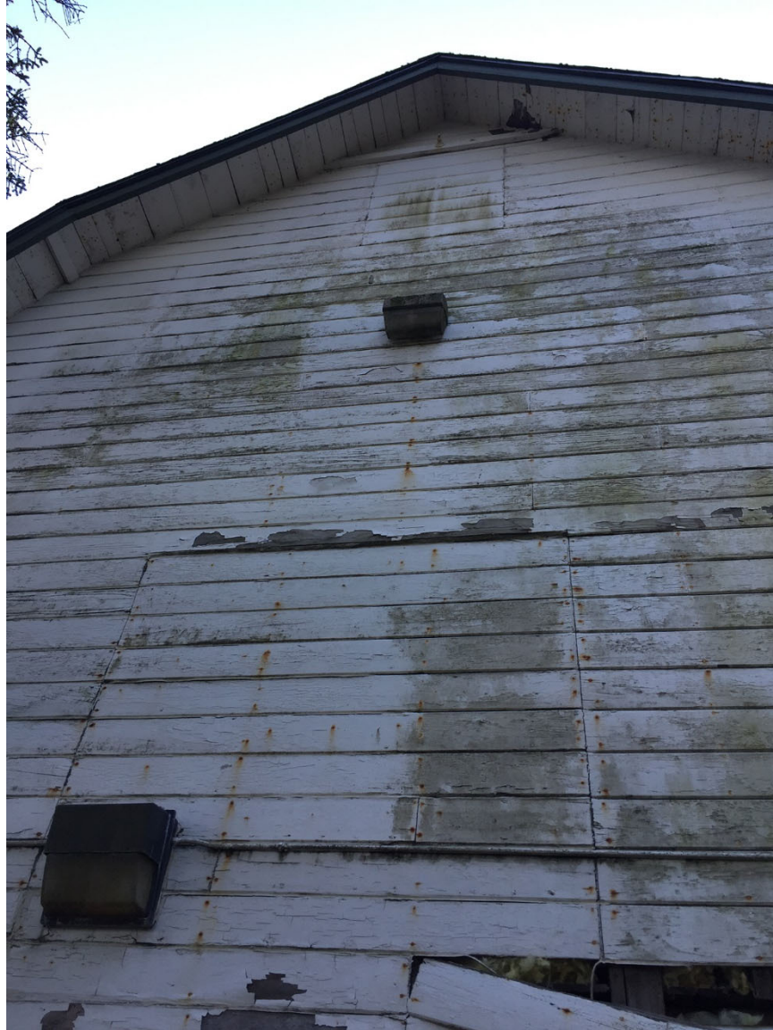
Photo 5: Detail of the east elevation. This photograph illustrates the various openings in the building which served the barn during its period of significance (1922-1931). Restoring these openings as windows or per the historic precedent is encouraged.
