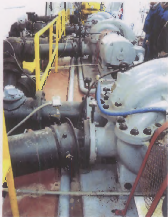
High Capacity Pumps and Piping
