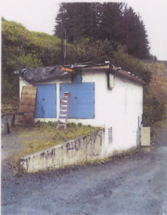
Monashka Pump House
