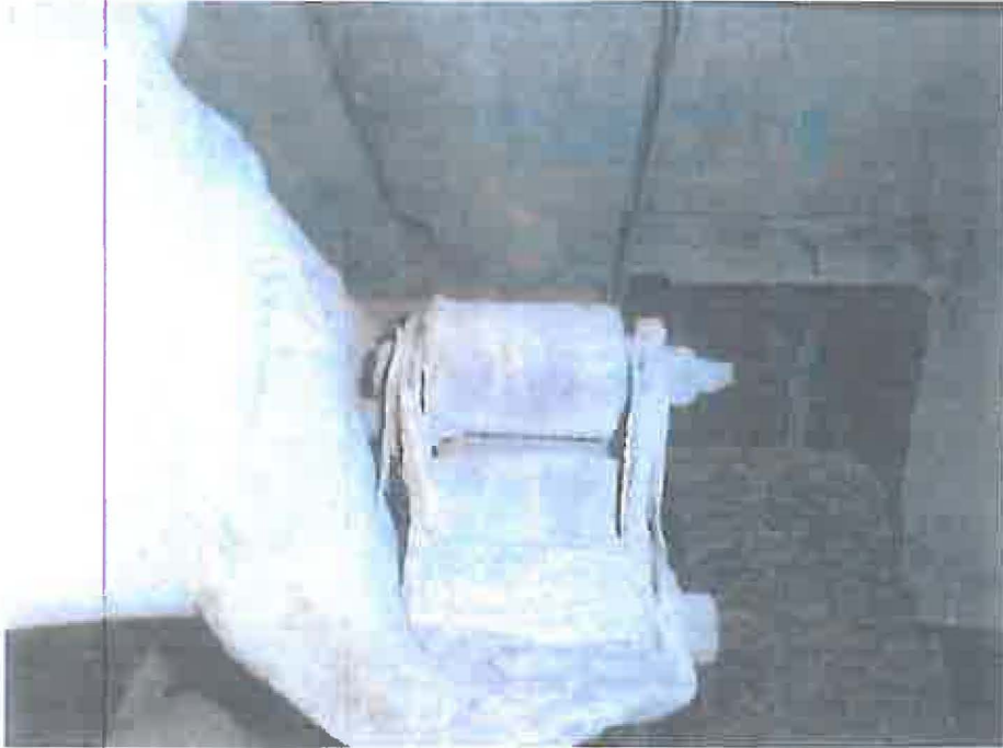
Condition of leaf springs, frame and shackles.
