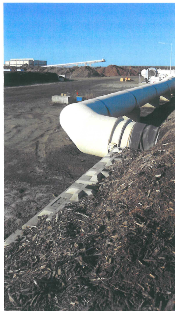
South Kern, California — aerated static pile composting with biofiltration of process air.
