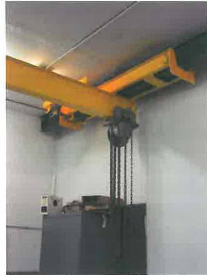
Crane end truck and 2-ton trolley hoist
