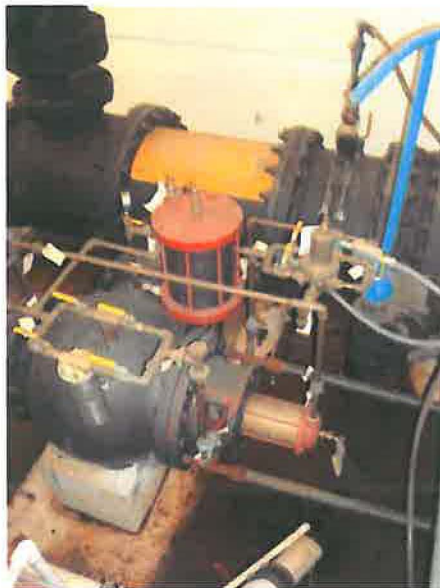
Surge relief valve
