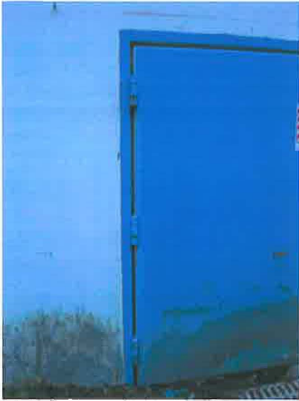
Water damage at wall and door
