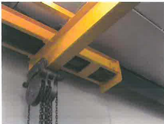
Bridge beam and underhung hoist
