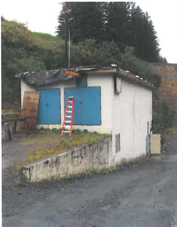
Monashka Pump House
