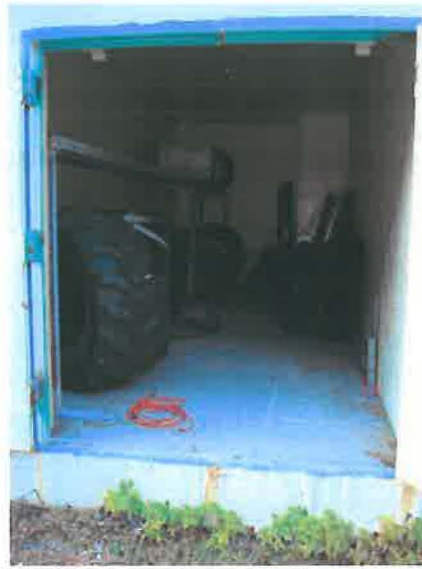
Double door at Fluoride Storage Room
