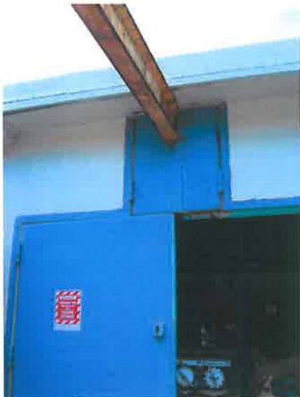
Crane rail at Container Storage Room
