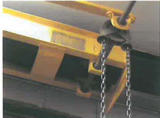
Bridge crane end-truck
