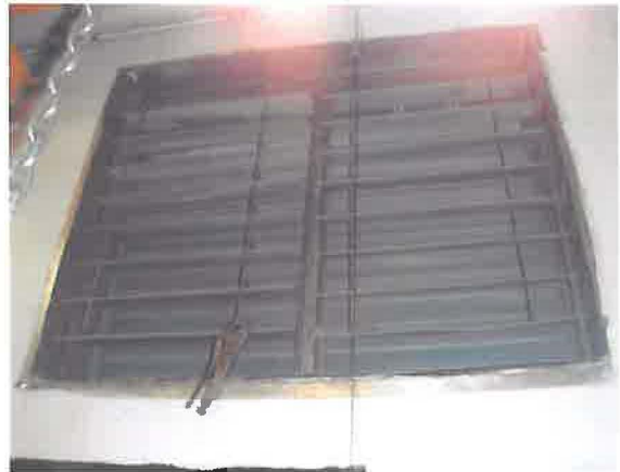
Existing damper in Machine Hall
