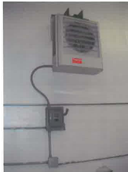
Unit heater in Machine Hall
