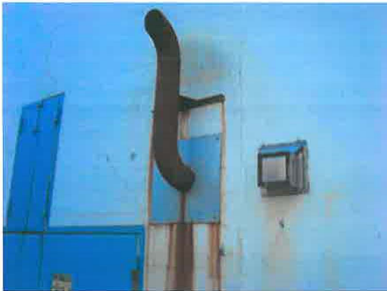
Machine Hall door and engine exhaust and furnace exhaust (right)
