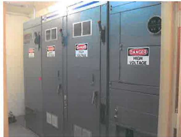
Main distribution panel with large motor starters
