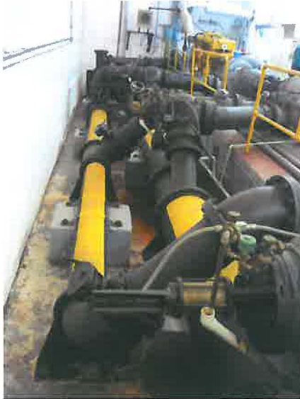
Suction and discharge piping
