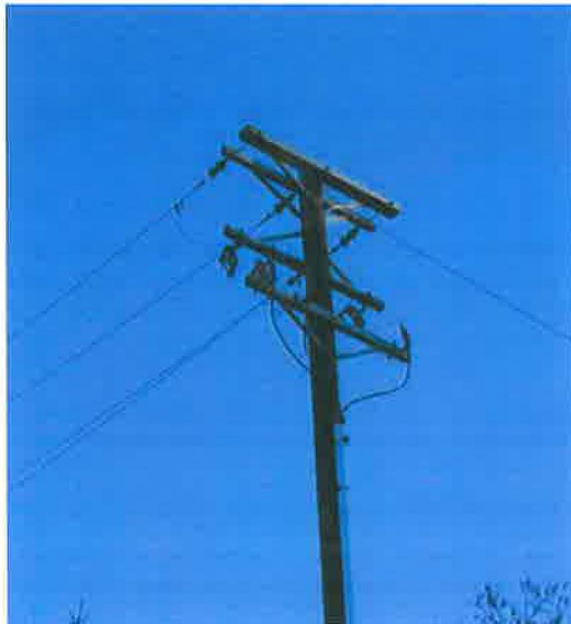
Utility 15-kVa riser pole feeding Pump House
