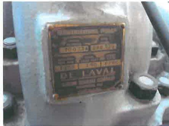
Pump No. 3 nameplate
