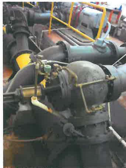
Pump No. 2 hydraulic check valve
