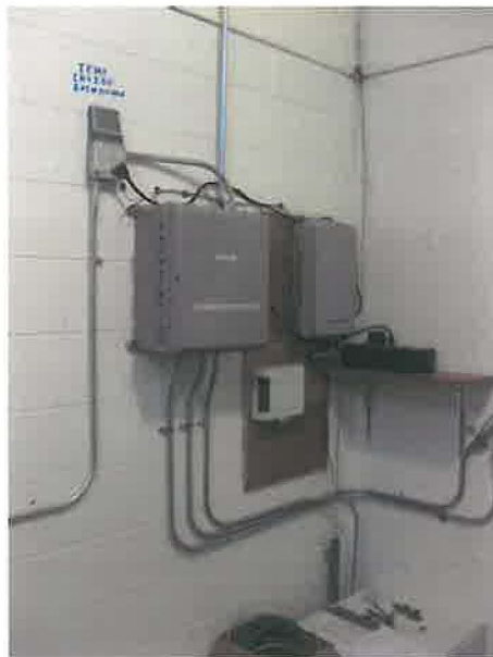
Existing I&C control panel and communications system
