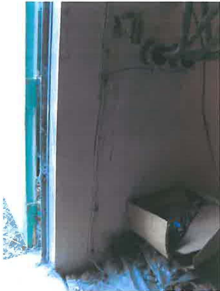
Grounding connections in KEA Room
