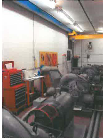
Motor drives and pumps
