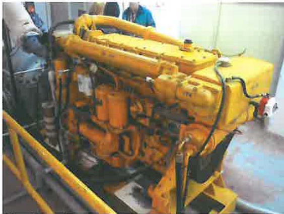
Diesel engine pump driver
