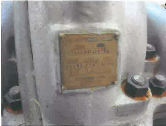
Pump No. 1 nameplate
