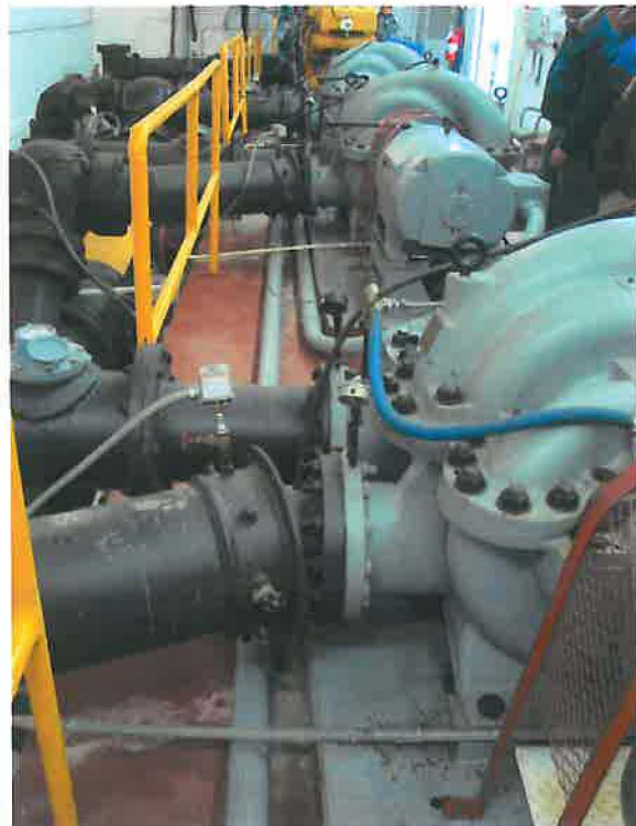
High Capacity Pumps and Piping
