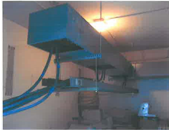
KEA Room bus duct with exposed energized bus
