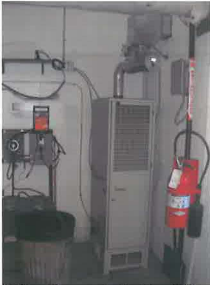
Oil-fired furnace in Machine Hall
