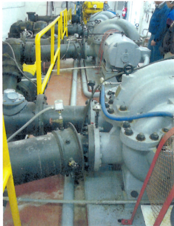
Photo of the Original High Capacity Pumps that Remain in Service
