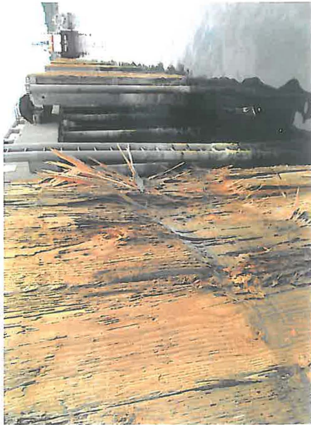
Pier 2, Kennicott Damage 7-24-11
