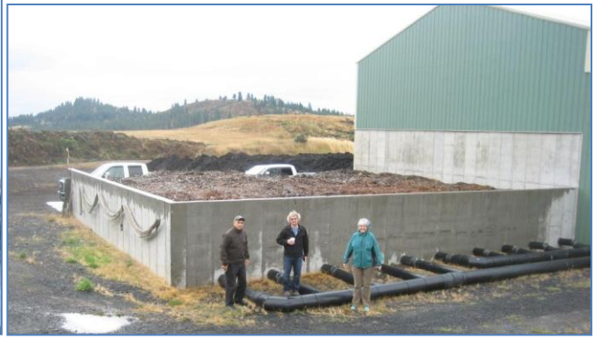
Figure 2 - Biofilter for Effective Odor Control
