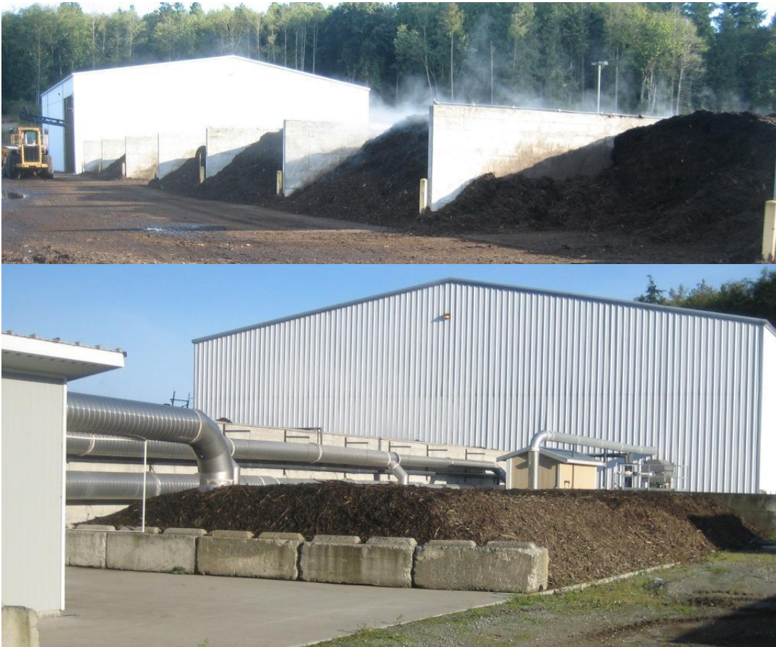
Figures 11-12 – ECS supplied Compost Bunkers and Biofilter System
