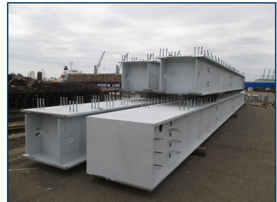
Box beams for grids P25 and P26 waiting for fit-ups in yard.
