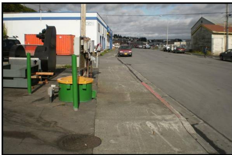
Figure 2: Lift Station 1 along Shelikof Street
