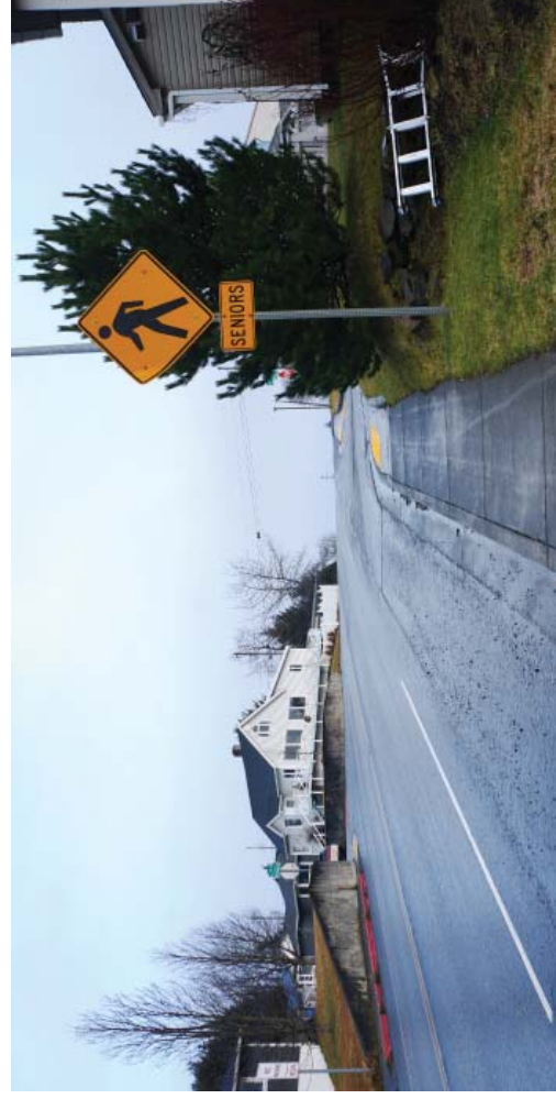
Image 27: As noted in the "Other Comments" row there is a pedestrian sign for crossing Rezanof Drive at the intersection of Mill Bay Road. But as seen in this image the crest in the hill above this crossing makes it hard to see oncoming traffic.
