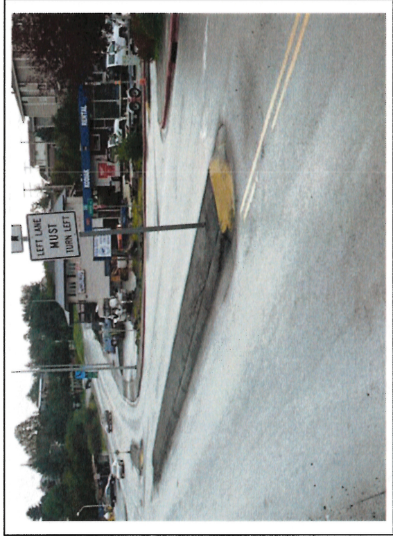
Photo 28 Looking at raised median and pavement that will be replaced by project from Sta. 507+00
