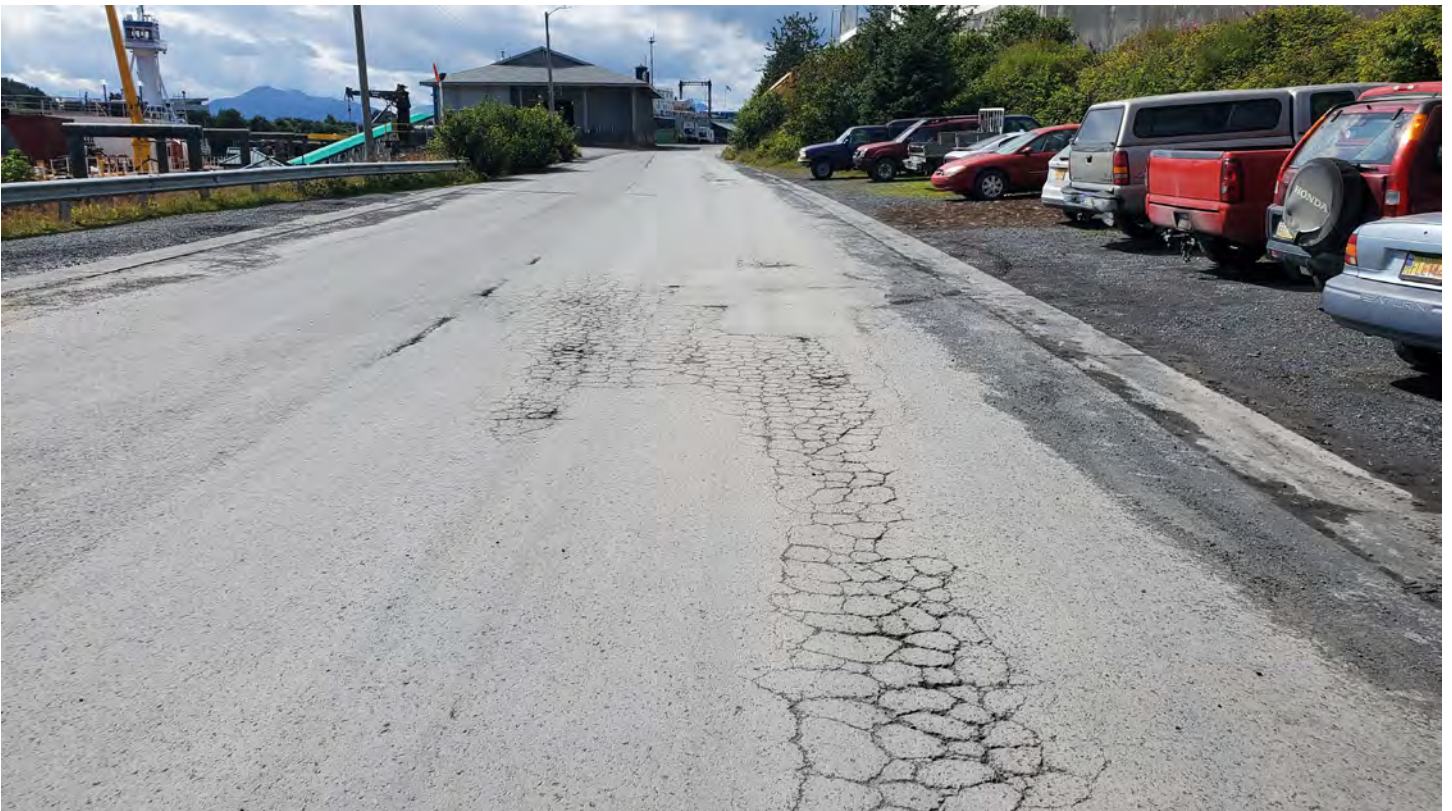
East Marine Way (cracking)
