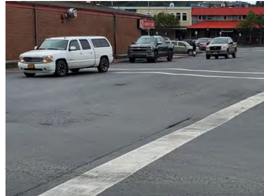
Rutting and pavement deterioration along West Marine Way, 2021
