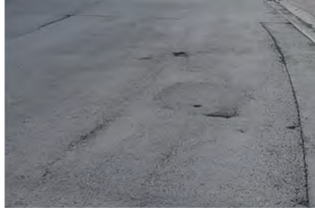
Pavement condition of Shelikof Street, 2021
