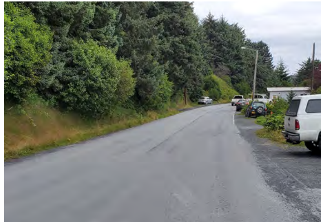
Mission Road, narrow lanes, no pedestrian path, and pavement cracking, 2021
