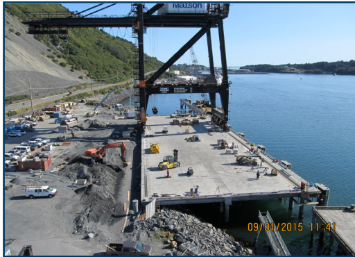
Overall view of site with Matson 100 gauge crane set in place on crane rails.
