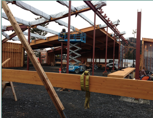
Contractor erecting glu-lams to support the library roof. View from main corridor looking toward stacks.
