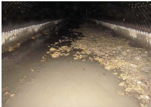
Photo 8 - Drain B – Rocky invert debris
