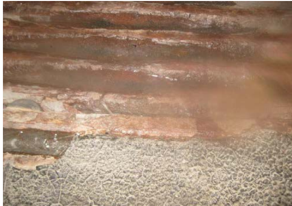
Photo 13 - Drain B – outlet has lost some coating and is corroded. Needs to be cleaned and recoated
