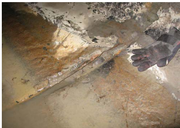
Photo 14 - Drain B – One of two infiltrating joints that needs to be sealed and recoated
