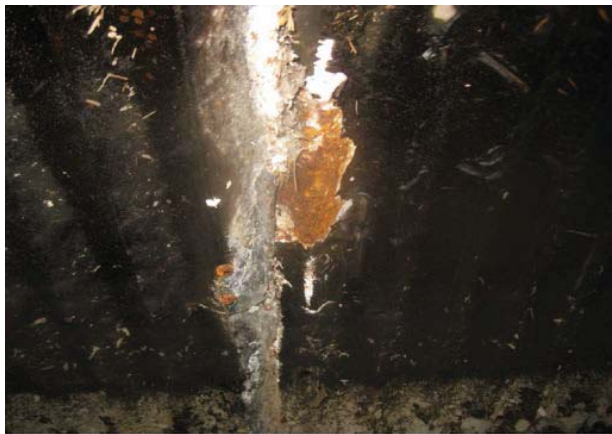
Photo 5 - Drain A – occasional flaking off of coating with minor Corrosion
