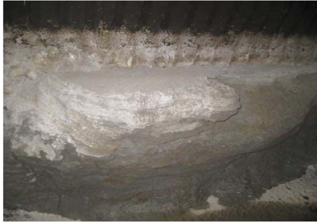
Photo 3 - Drain A – typical 10" deep silt/sand deposit
