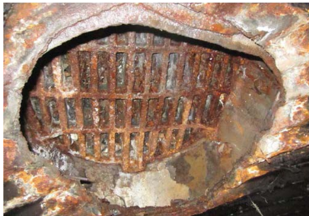
Photo 11 - Drain B – Flame cut manhole opening with serious Corrosion needs to be cleaned and recoated
