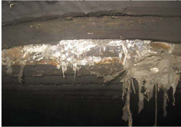
Photo 4 - Drain A – Joint with 1" separation and 1-1/2" offset
