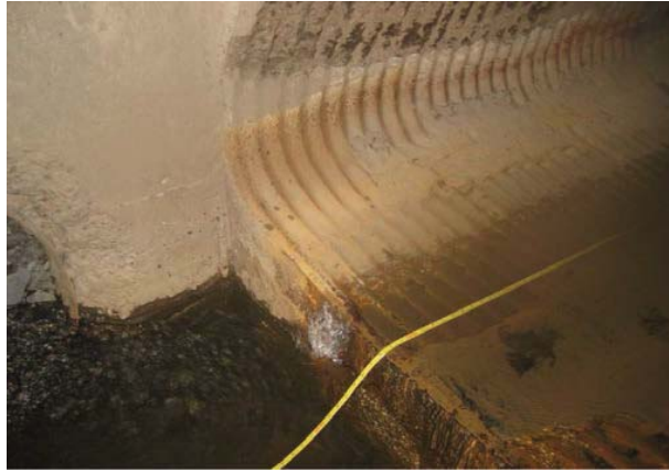
Photo 6 - Drain A – Outlet steel is exposed and needs to be cleaned and recoated
