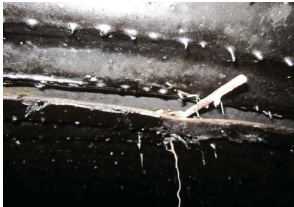
Photo 10 - Drain B – Separated joint with 1” offset
