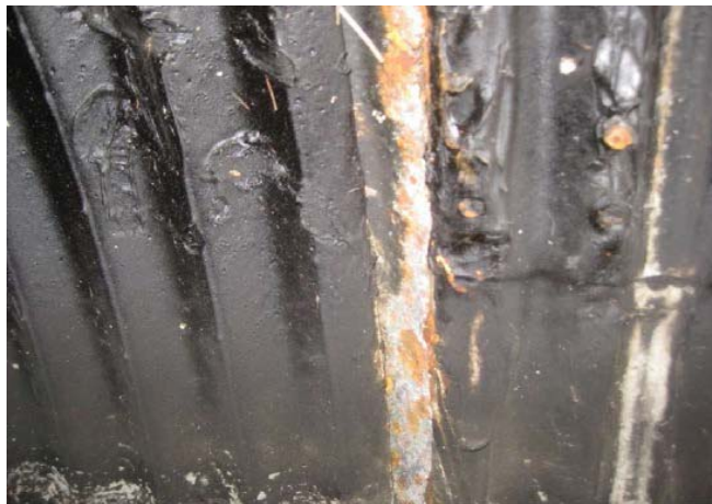
Photo 2 - Drain A – Separated joint showing minor incipient corrosion
