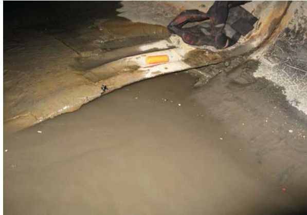
Photo 12 - Drain B – 12" horizontal void that needs to be filled
