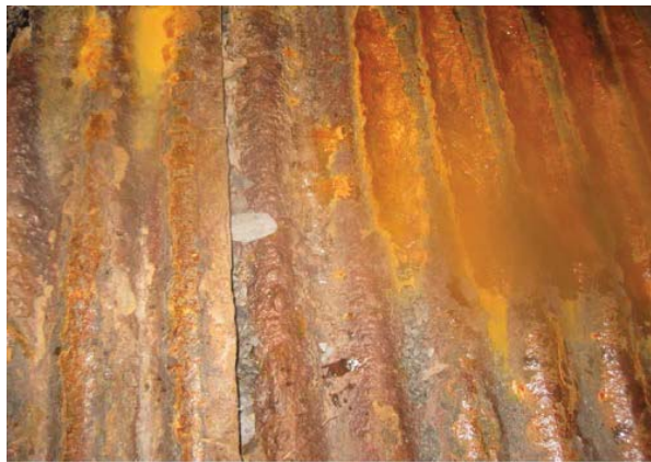
Photo 7 - Drain A - Corroded outlet where coating is missing
