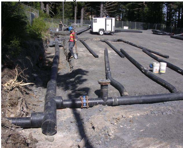
EXHIBIT 2 Compost Aeration Piping
